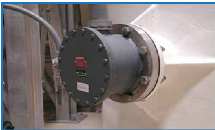
RO CIP Tank Heater
