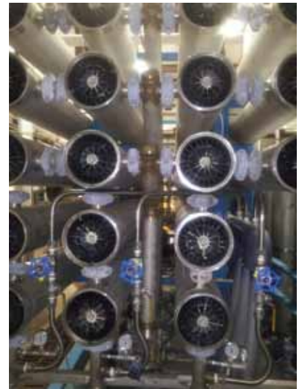
Reconfigured Skid showing central distribution headers to inlet of 1st Stage pressure vessels (Note that the each vessel was rotated 90 degrees to align to header)
